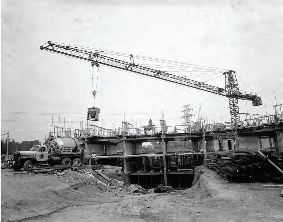
Figure 4.6. This photograph depicts handset-form method construction being used on a housing project in 1964. Unlike flying forms, traditional methods require the scaffolding and formwork to be disassembled and reassembled manually. The climbing crane delivered materials and had not yet been employed in the hoisting of large flying form sections. [Source: City of Toronto Archives.]
