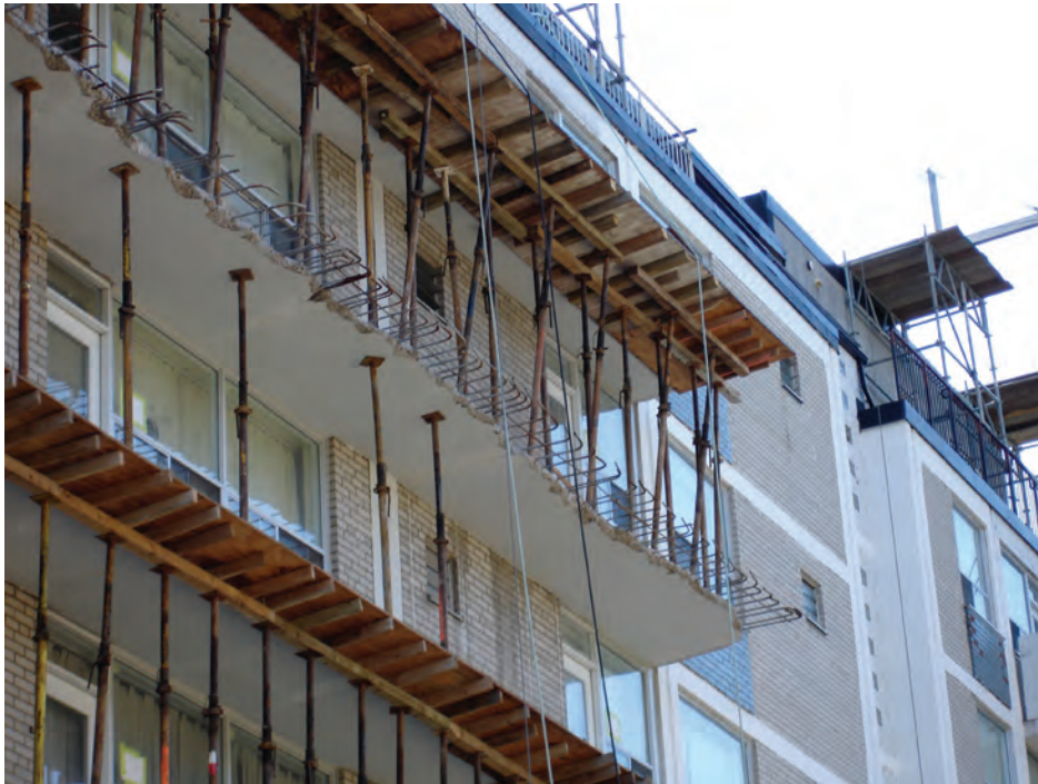
Figure 8.19. Deterioration of essential components of tower buildings can lead to the need for costly repairs and replacement. Some of these repairs, such as balcony restoration, are expensive and do not have a payback since the energy and water conservation of the building has not been improved.
