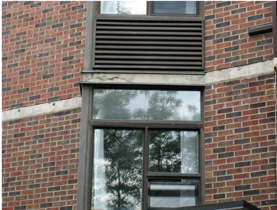
Figure 5.3. Photographs of the deficiencies are important for documentation purposes. The deteriorated exposed slab edge depicted above must be properly repaired prior to overcladding. Design details for the integration of existing grilles with the overcladding may begin to be investigated. [Photo: Halsall Associates Ltd.]
