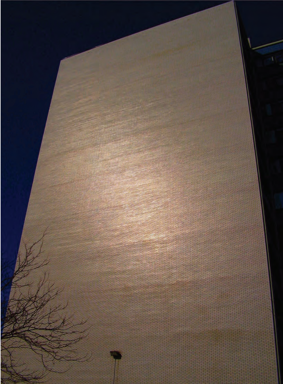
Figure 3.1. A brick clad shear wall without any window openings represents the lowest cost existing condition of the substrate for adequately supporting the new façade, and the cost of the materials selected for the overcladding. Repairs to the existing envelope may prove expensive, and durable materials with a high aesthetic appeal will further add to this cost. Retrofitting south-facing walls of this kind with photovoltaic and/or solar thermal panels will yield the lowest life cycle costs, and eventually revenue generation. [Photo: faculty x.]
