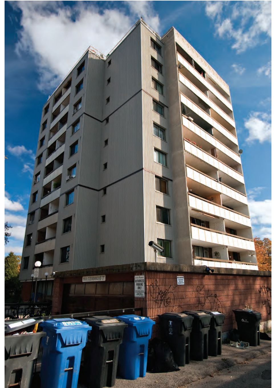
Figure 7.1. An example of a cosmetic retrofit that does not address building system integration opportunities. Regrettably, neither the durability nor the energy efficiency of the balconies has improved. [Photo: Jesse Colin Jackson.]
