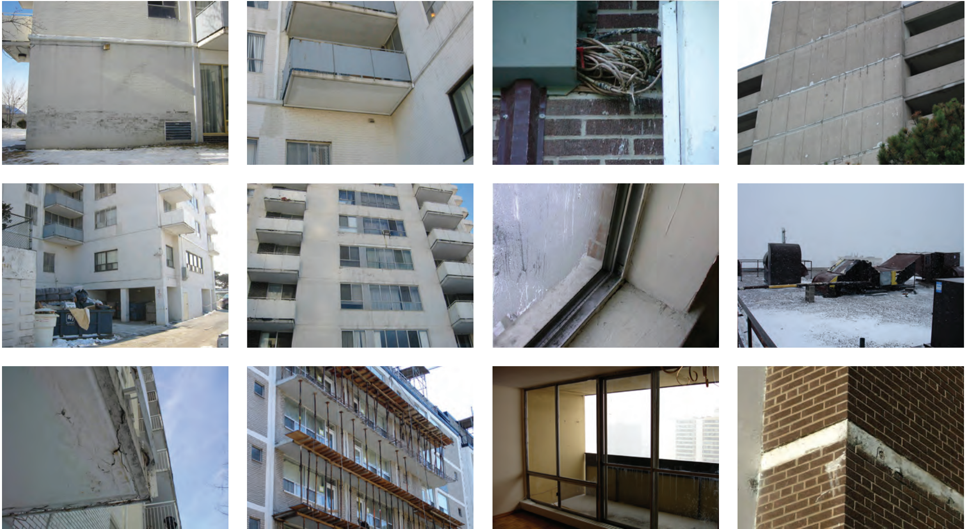
Figure 4.15. Deterioration and obsolescence are commonplace in tower apartment buildings. The aging tower apartment stock has a pathology that reflects its common design and construction characteristics. Most prevalent are cladding failures and deterioration of cantilevered balcony slabs. Failure of cladding at grade due to uncontrolled moisture migration is widespread. Windows are typically leaky, exhibit poor thermal performance and in some cases, deterioration of the frames and sashes. Exposed concrete elements are beginning to reveal the onset of carbonation and the corrosion of reinforcing steel, in many cases leading to spalling of the concrete surface. Mechanical equipment is often obsolete and in poor condition, especially exposed equipment and ductwork located on rooftops. The major building services are often nearing the end of service life. Piping has deteriorated and its thickness has eroded over time. Ductwork is sound but requires thorough cleaning. Electrical wiring is normally serviceable, but cabling for television, telephones and telecommunications has spiraled into chaotic disorder and makeshift adaptation to ever changing tenant preferences and technological advances. Elevators, the lifeblood of high-rise apartment buildings, are typically in need of rehabilitation and their lack of reliability is frustrating to tenants who are pressed for time in meeting the demands of modern urban lifestyles.
