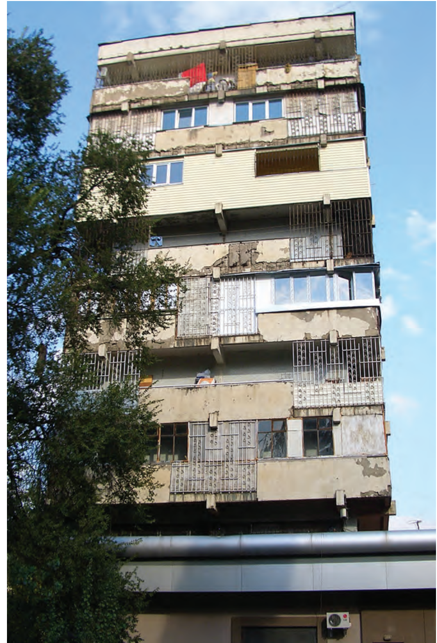
Figure 2.3. Apartment blocks like this one, situated in the former Soviet Union, teach important lessons about coordinated renewal strategies. Each floor of this building has been addressed individually by its inhabitants in a makeshift manner that has not improved durability or energy efficiency, and has also failed to enhance architectural aesthetics. This extreme example underscores the need for architectural standards developed in support of tower renewal. [Photo: V. Menkov]
