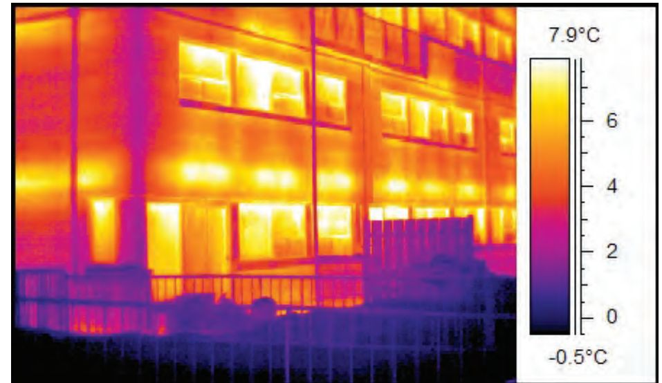
Figure 5.11. The baseboard heaters beneath the second storey windows are evident in this thermographic image. Much of the heating in tower buildings travels directly to the outside without improving thermal comfort in the living spaces. [Image: Boldstar Infrared Services Inc.]
