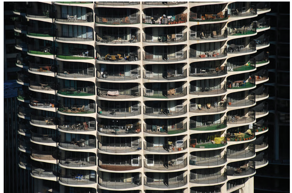
Figure 3.2. The cooperation of tower occupants for the removal of personal possessions and furniture from balconies is an important factor influencing the timely execution of retrofit work. Retrofit cost premiums may be compounded when an unusual geometry is combined with a high occupancy of balconies. [Photo: SolarWind – Chicago.]
