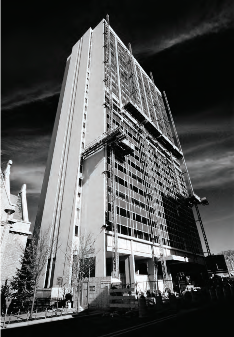
Figure 3.9. The front façade of a tower retrofit is approaching completion. Note the deployment of climbing mast work platforms and their configuration to access the shear walls. The staging work area impinges on the street and requires special permits and procedures for pedestrian and vehicular traffic control. [Photo: Gary Easter.]
