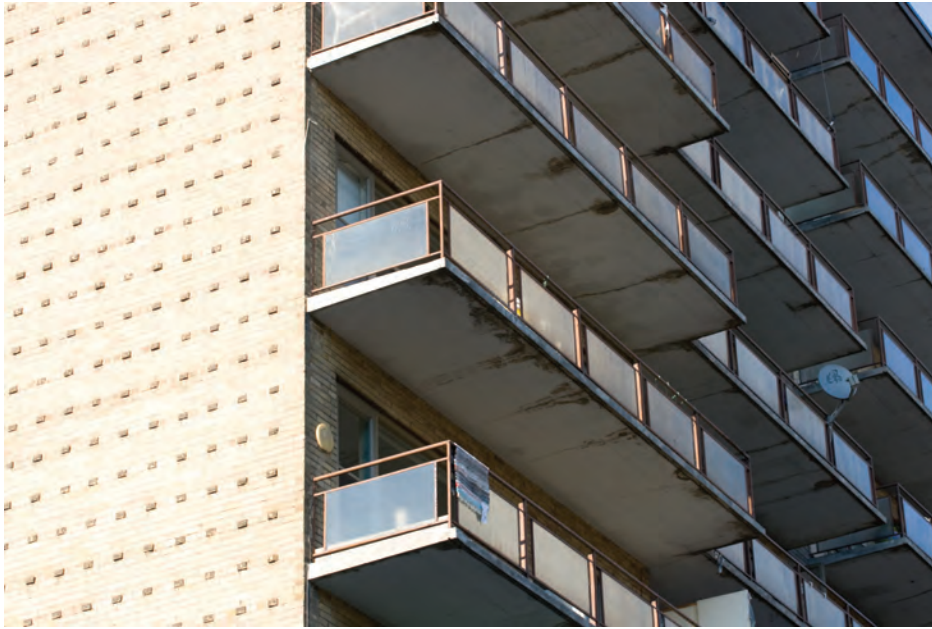
Figure 7.27. Exposed balcony slabs are the weak link in the existing stock of tower buildings. [Photo: Jesse Colin Jackson.]
