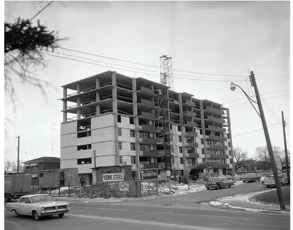
Figure 4.5. By the mid-1960s the reinforced concrete frame became the system of choice for mid-rise apartment buildings, like the one depicted above, as well as high-rise towers. The floor slabs are visibly exposed on the end walls because the infill masonry envelope spans from top of floor slab to underside of floor slab. Articulated canopies over the front entrance were common features. [Source: City of Toronto Archives.]
