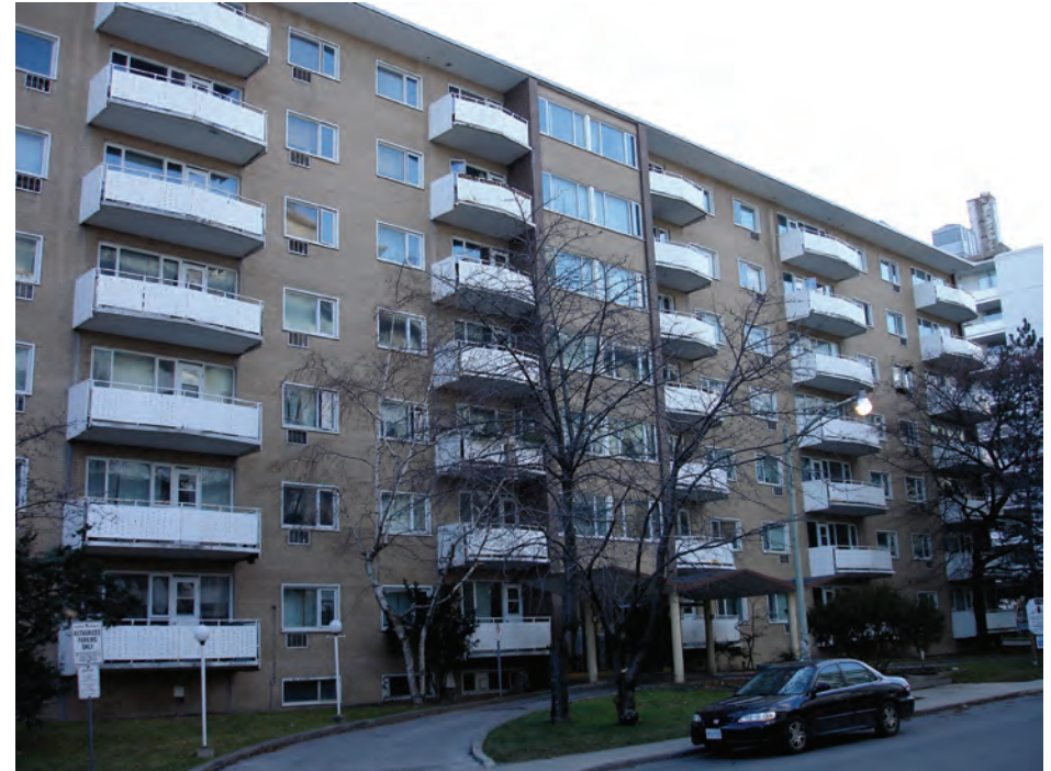
Figure 7.37. There are two types of balconies on this apartment building. The centrally located balconies serve one suite and have one side enclosed by the projecting shear wall. The flanking balconies each serve one suite but are open on all sides. Special consideration must be given to the packages terminal air conditioning (PTAC) units located beneath the windows when designing the overcladding. Thermal bridging, future replacements of the PTAC units and management of the condensate dripping from the units when they are cooling the suites are among the chief concerns.
