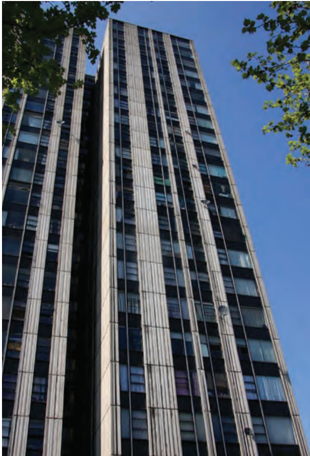
An example of a typical tower apartment building prior to retrofit. Evidence of water damage is visible on the concrete façade elements.
