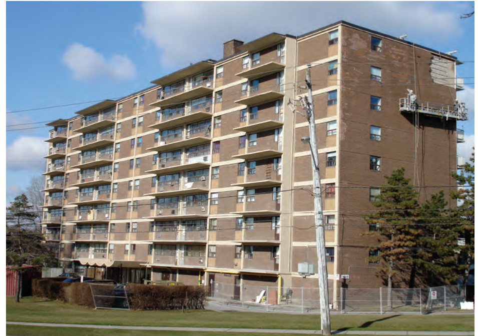
Figure 4.16. This 1960s apartment building is undergoing a major repair to the balconies and brick cladding that may have been largely avoidable if better maintenance practices were adopted. Again, there is no payback in these rehabilitation measures.
