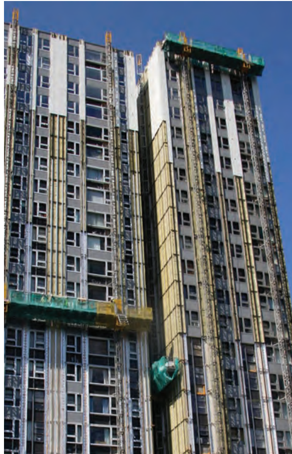
Retrofit work proceeds in stages from the top down to avoid damage to finished elements from falling debris. Note the deployment of climbing mast work platforms.
