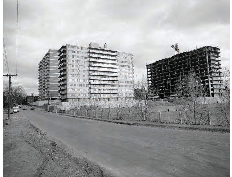
Figure 4.7. Concrete tower construction at Roselawn Avenue and Chaplin Crescent in Toronto. Aided by flying form technology, developers were able to “mass produce” housing with robust building armatures in response to Toronto’s explosive population growth. In Canada’s large urban centres, starting towards the early 1960s, concrete flying form technology was being invented. Reinforced concrete tower buildings were the ideal test bed for the technology, featuring repeated floor plans that could be sequentially erected one floor after another. To reduce labour costs, an aluminum framing system supported formwork that could be slid out sideways by the climbing crane after the concrete was set, and lifted in place on the next floor. The greatest economy was achieved when the floor plans were simplified and the building layout rendered symmetrical. Standardized dimensions were derived from a modular corresponding to Canadian lumber and plywood sizes to minimize cutting and waste. This highly rationalized system of construction was in reality a vertical assembly line that manufactured housing no differently than so many products manufactured in other sectors of the economy, such as automobiles and appliances. [Source: City of Toronto Archives]
