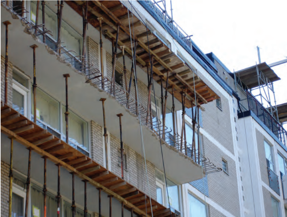
Figure 4.13. Carbonation is the leading cause of balcony slab edge deterioration. The cost of repairs is relatively expensive because new guards are also usually installed. This type of necessary structural repair has no payback. Encapsulation of the concrete by overcladding or balcony enclosure is a preventive measure with payback due to energy savings.
