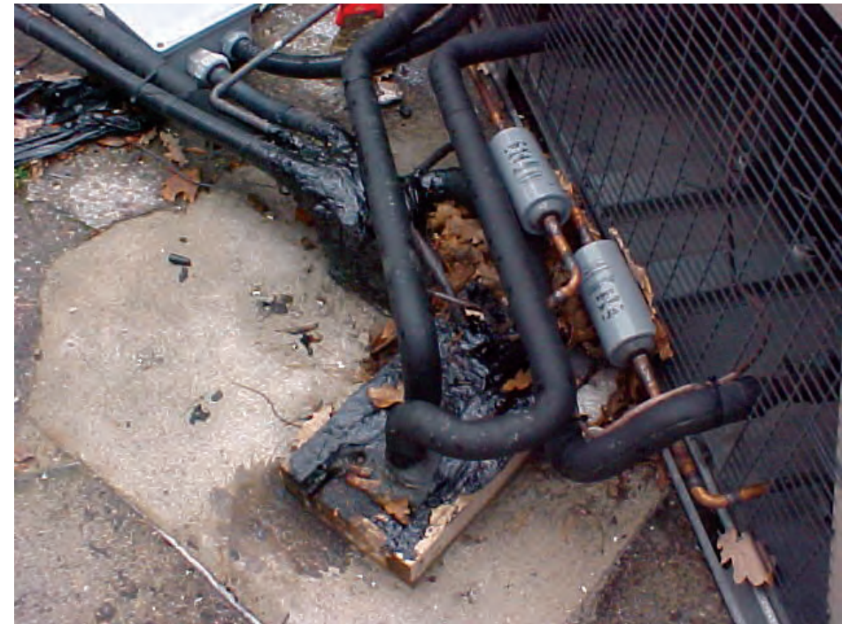
Figure 5.5. The service condition of the air-conditioning tubing depicted above is fair, but the penetration through the roofing system has not been properly addressed. This opportunity arises with roofing replacement where more appropriate measures may be employed, rather than relying on large quantities of caulking. [Photo: J. McBride and Sons Ltd.]
