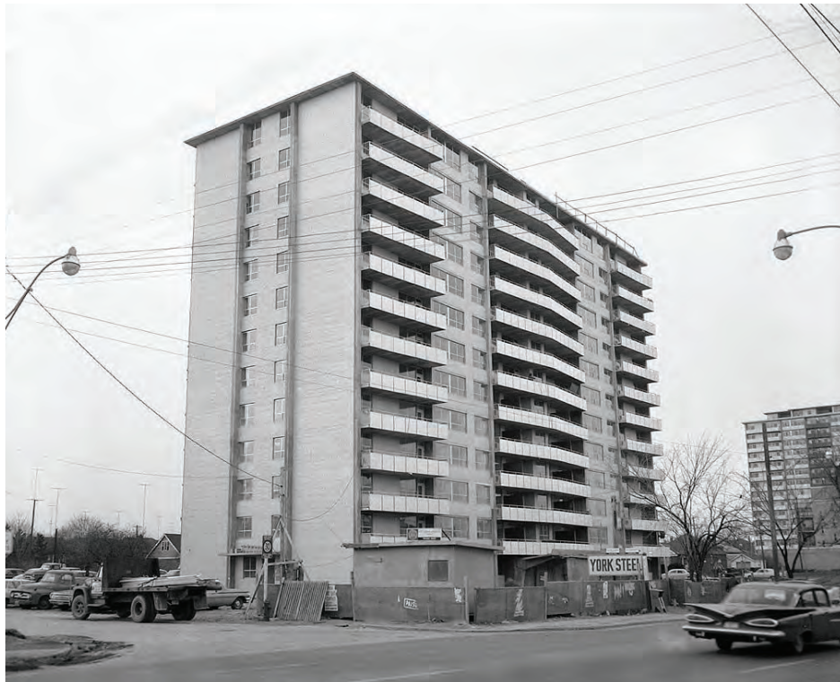
Figure 4.12. A typical tower apartment building of the 1960s nearing completion. Many tower building owners lacked the sophistication to implement preventive maintenance practices, often assuming the selected materials were durable, “maintenance free” and made to last a lifetime.
